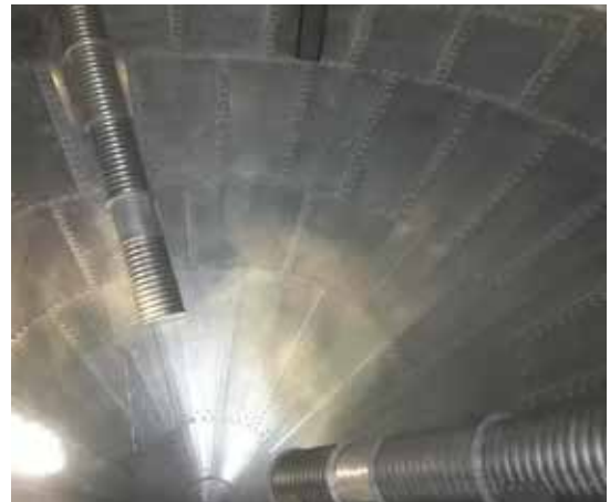
— Photo of hopper silo aeration ducts mounted on silo
