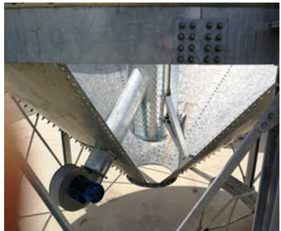
— Photo of hopper silo rocket aeration with centrifugal fan
